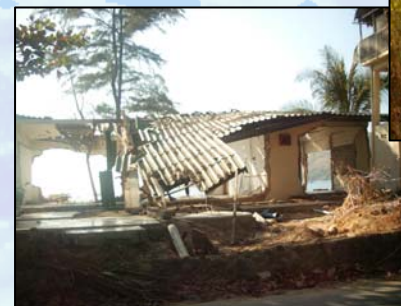
Nearby Tsunami damage
